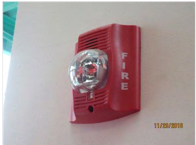
Fire Alarm Strobe
