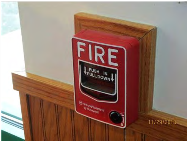
Fire Alarm Pull
