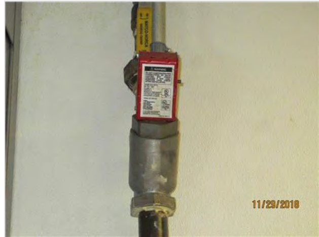
Automatic Fuel Shut Off
