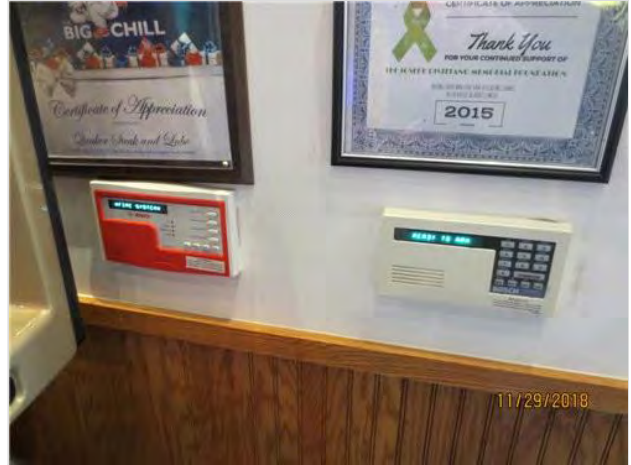
Burglar / Fire Alarm Keypads
