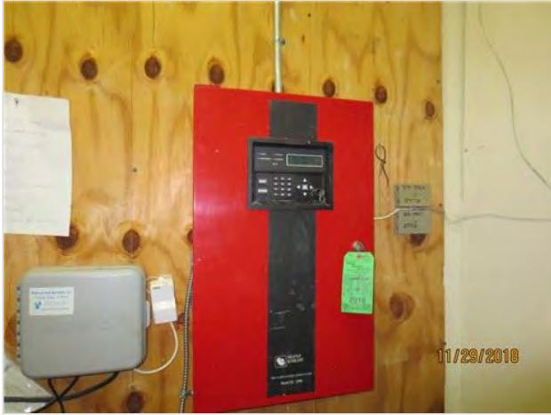
Fire Alarm Panel
