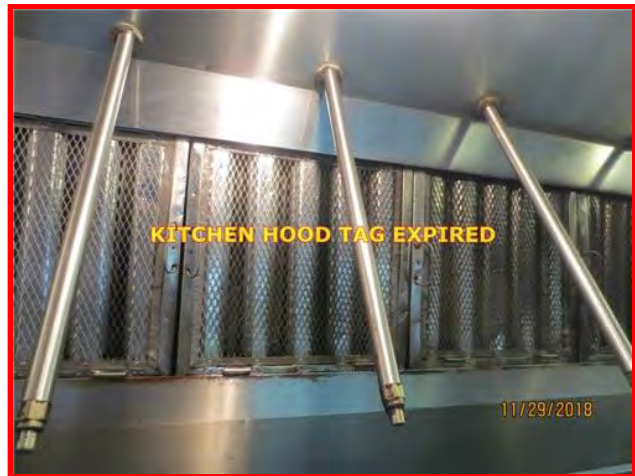
Hood / Baffles # 1 / EXPIRED Hood Tag
