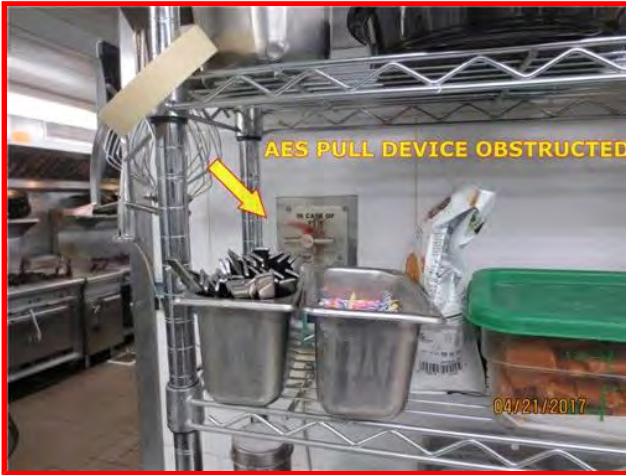
AES Pull # 1 / OBSTRUCTED
