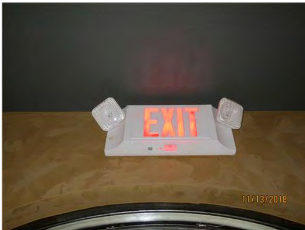
Emergency Exit Sign / Lighting
