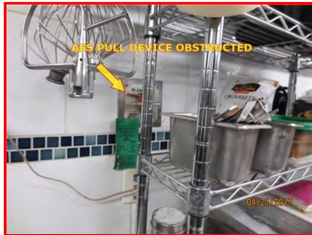
AES Pull # 1 / OBSTRUCTED
